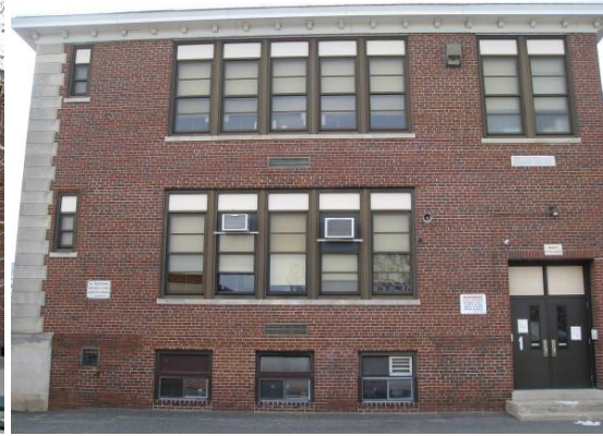
Unsealed window air conditioning units
