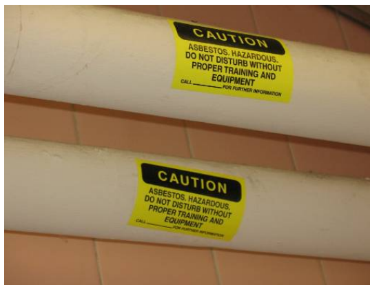
Asbestos Warning on water pipes
