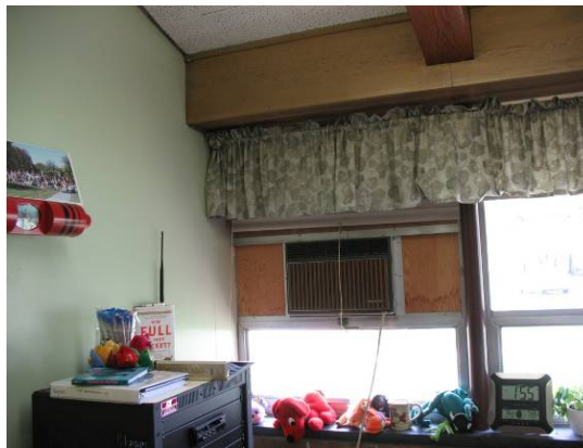
Older window air conditioning unit
