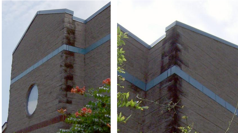
Signs of water runoff from faulty roof cap flashing seams.
