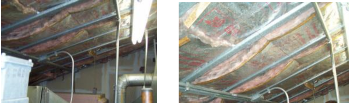
Roof insulation in attic attached directly on underside of sheathing with no specified airspace for air to circulate between sheathing and insulation.
