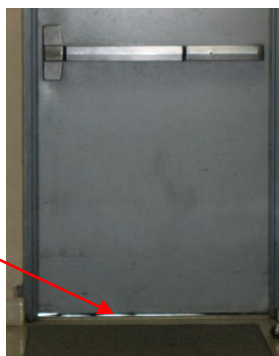
Missing or worn weather-stripping at door (typ.)
