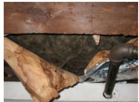
Defective Fiberglass Insulation under Main Floor
