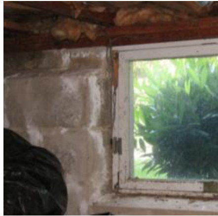
Signs of Water Penetration on Updated Foundation Walls
