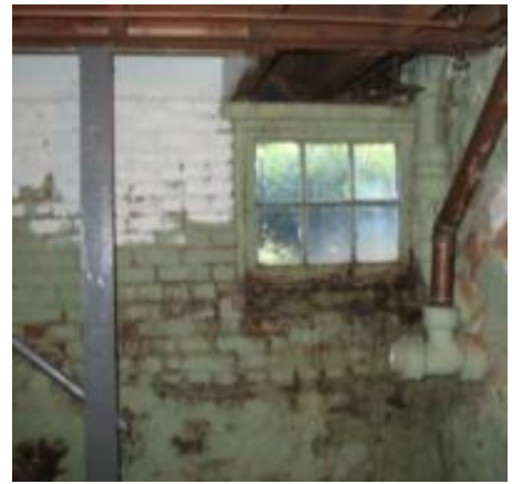
Signs of Water Penetration on Original Foundation Walls
