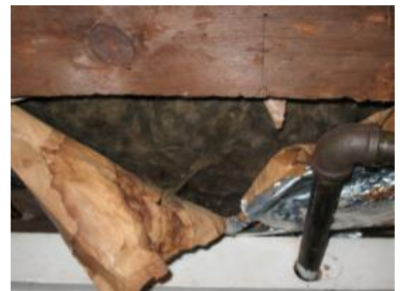
Defective Fiberglass Insulation under Main Floor
