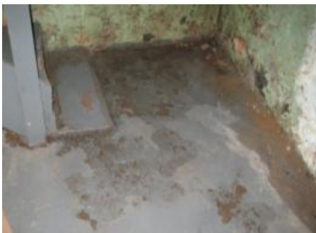
Water Penetrating from Basement Slab
