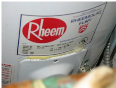
20 gallon water heater
