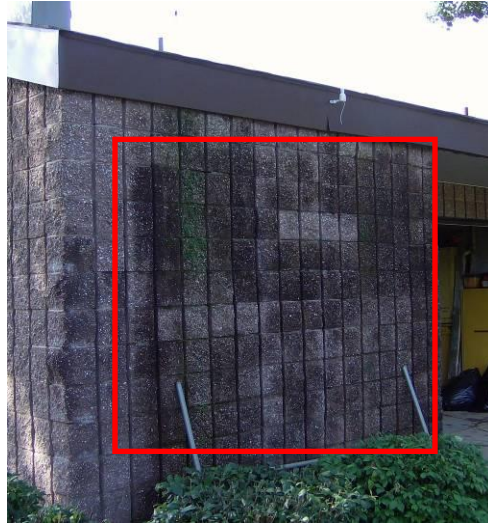
Water soaked wall due to lack of gutters or sufficient overhang
