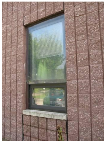
Fixed and casement windows with polycarbonate cover
