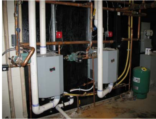
Two NTI high efficiency boilers
