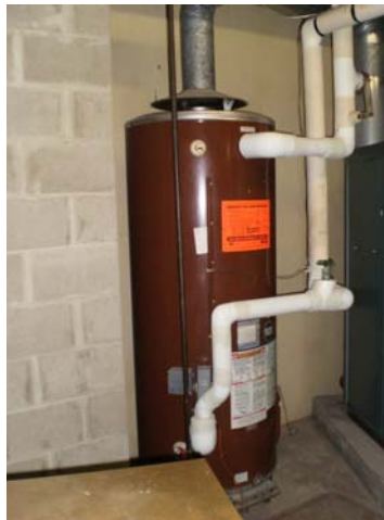
Hot Water Heater in Basement Mechanical Room
