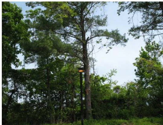
Exterior light left on during daytime hours
