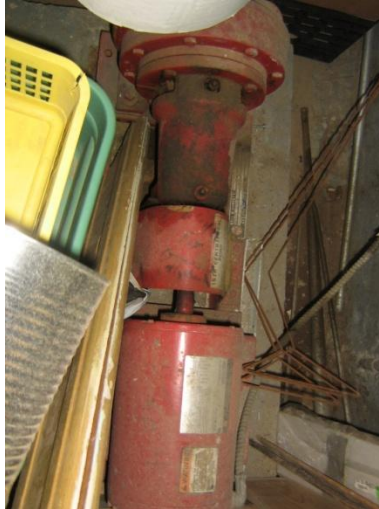
Heating system pump
