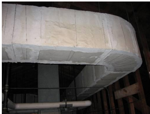
Asbestos on an unused Air Handler trunk in 1950 section of the building
