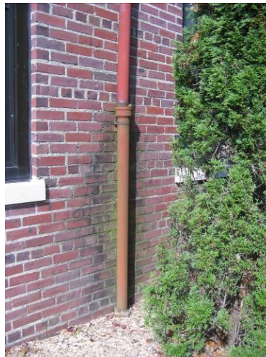
Signs of water damaged wall caused by leaking downspout connection
