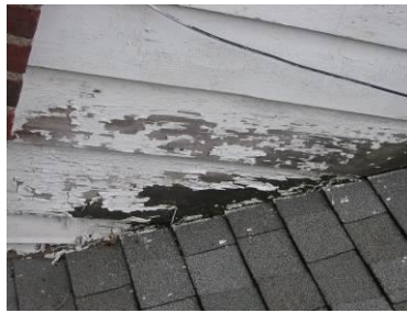
1996 asphalt roof section showing deterioration of siding
