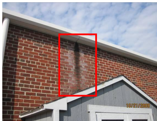
Water damaged wall section
