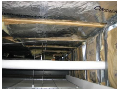
R-30 foil-faced fiberglass in plenum above Room 11
