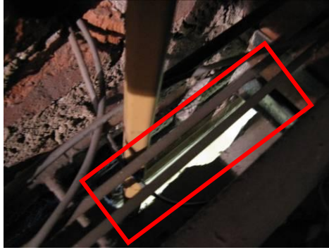
View from attic through large plumbing penetration to floor below
