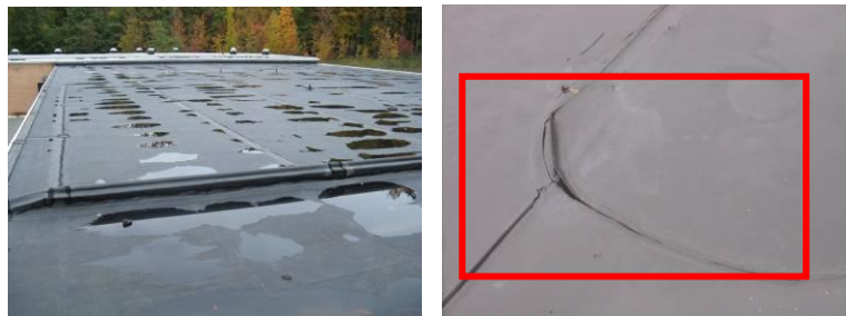
1990 EPDM roof showing pooling post rainfall; Un-sealed seam on same roof area
