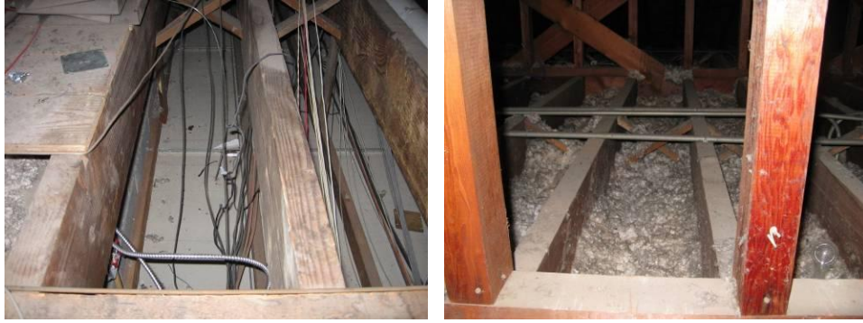
Open attic bays without insulation in 1950 section of building; approximately 1" blown insulation
