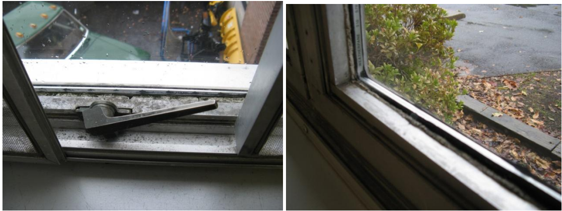
Older windows showing cracked and damaged caulk
