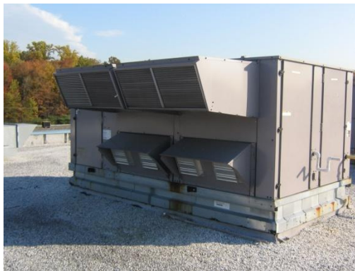
One of the two VAV Packaged Rooftop Units on the 2002 Addition
