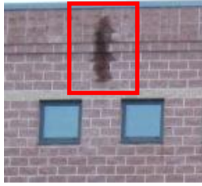
Uncontrolled roof water run-off
