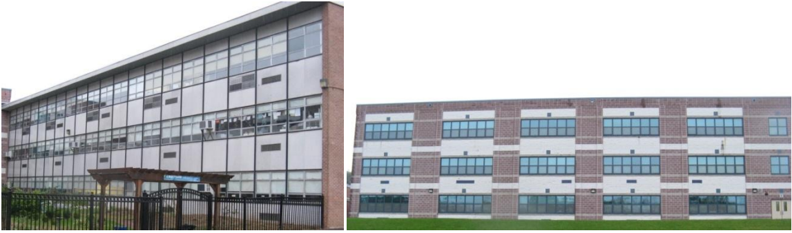
Older wall section with aluminum single pane windows; New addition with low-e double pane windows
