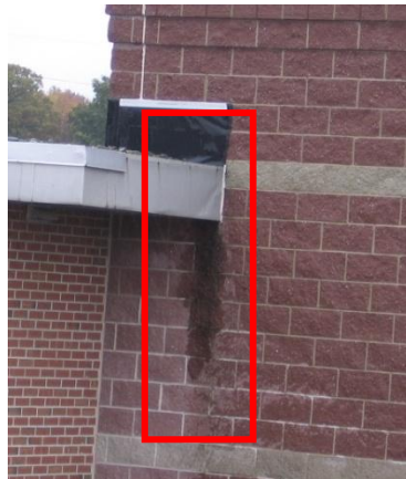
Roof water run-off causing water to penetrate exterior wall finish
