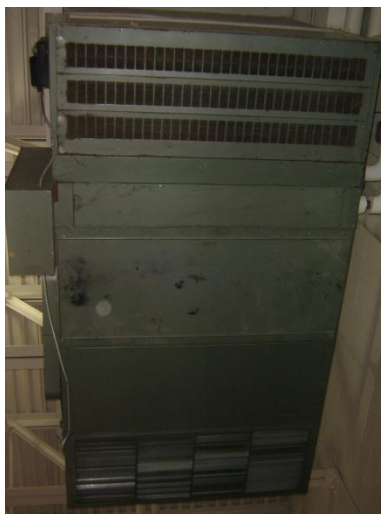
One of Four Heating & Ventilating Units Serving the Original Gym
