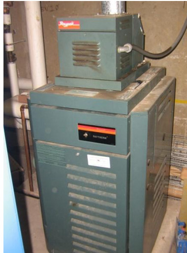
Domestic Water Heater
