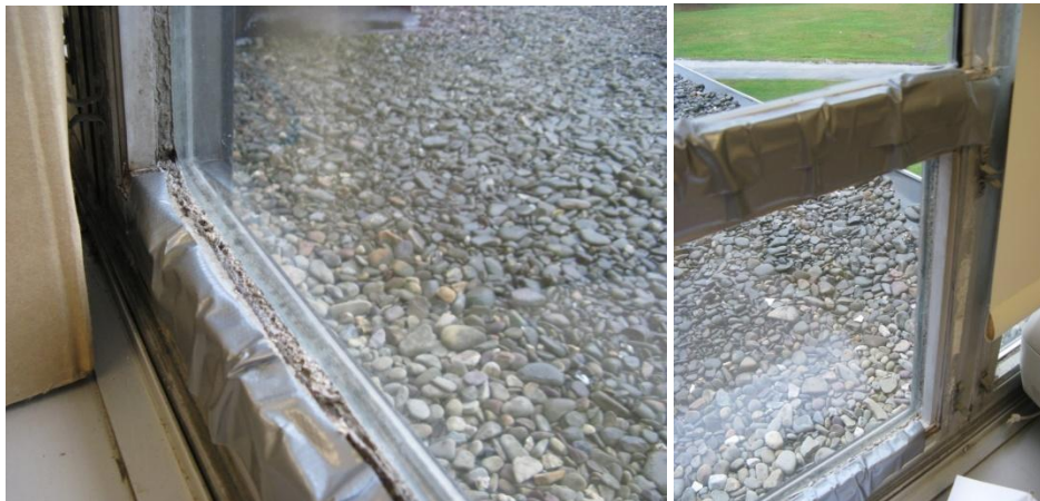
Duct tape used in classroom to try to prevent air infiltration
