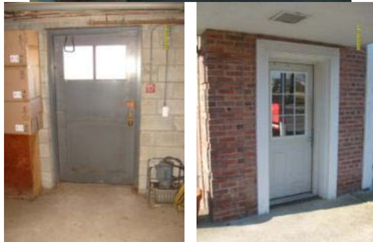
Missing/ worn weather stripping
