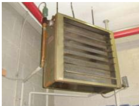
Unit heater in garage.
