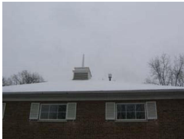
Vehicle exhaust duct up through roof
