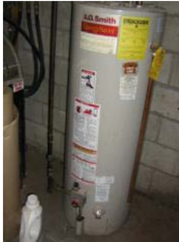
Domestic water heater
