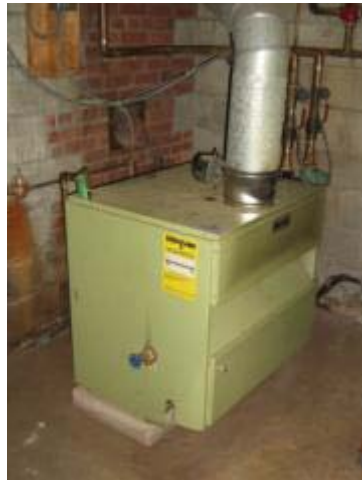
Gas fired boiler in lower level storage room
