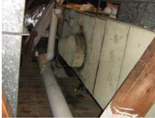
Air Handling Unit above stage area
