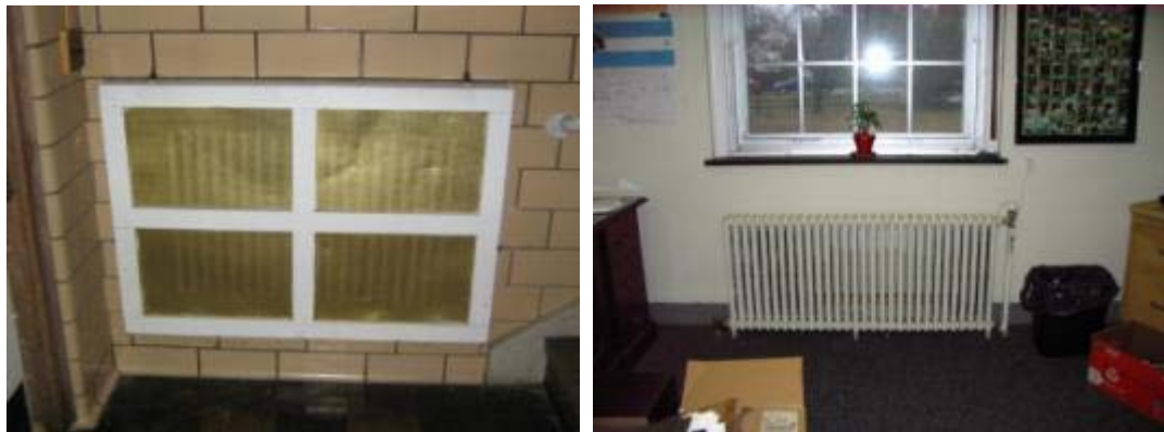
Typical radiators throughout the building
