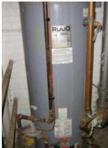
Domestic Hot Water heater
