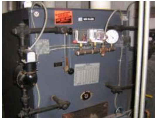
Gas fired boiler in Mechanical Room
