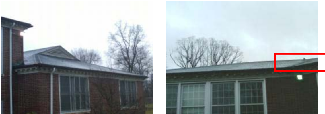
Missing/ ineffective flashing
