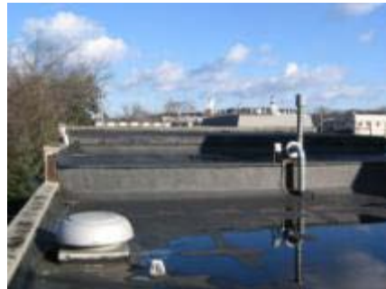
Exhaust fan (left) and vehicle exhaust (right, typical for (2)) on roof
