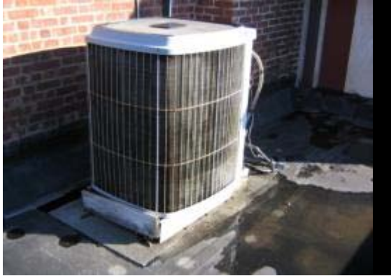
Split system condensing unit on roof
