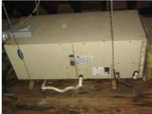
Split system air handler in attic
