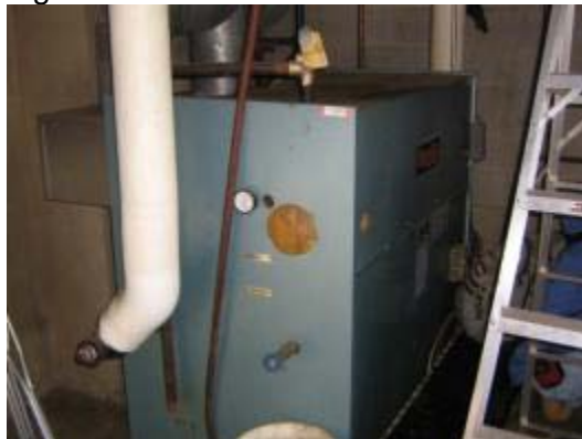
Gas fired boiler in Mechanical Room
