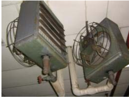
Unit heaters in garage
