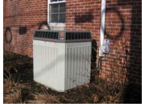
Split system condensing unit on grade
