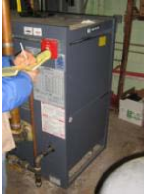
Gas-fired boiler in boiler room
