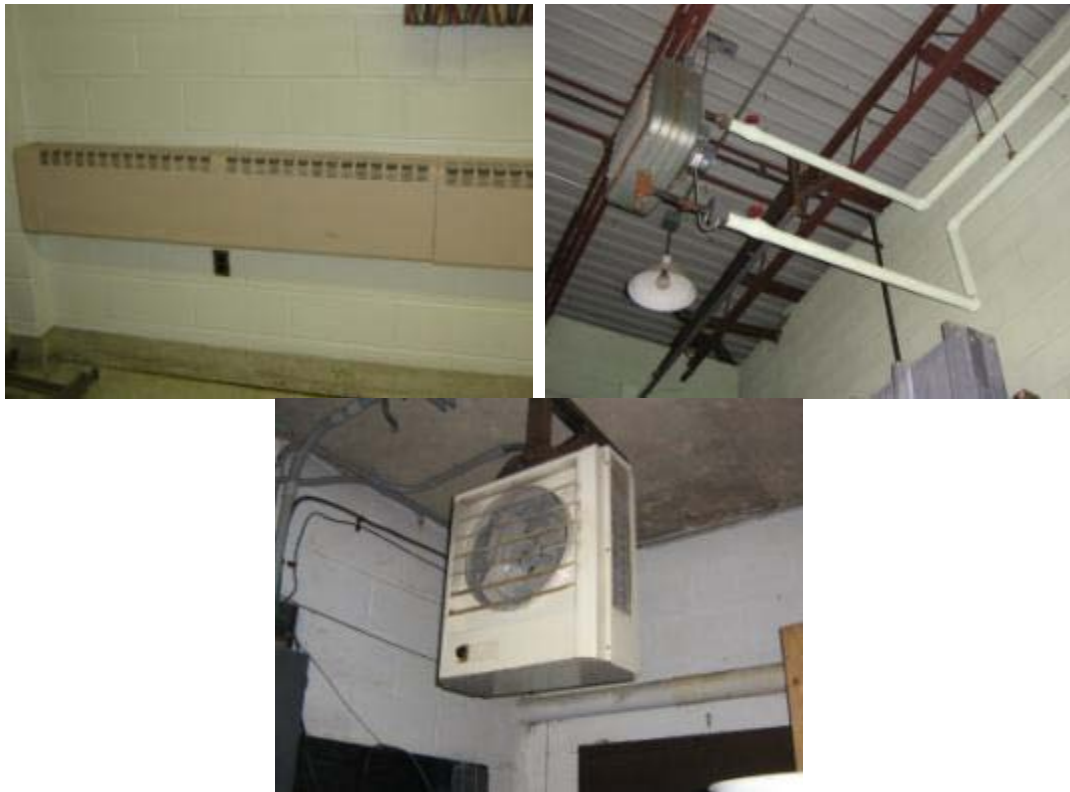
Radiators throughout the building, hydronic heaters in basement, and electric unit heater in pool's main pump house
