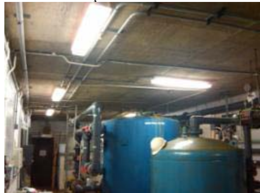
Underground Rear Pump Room
