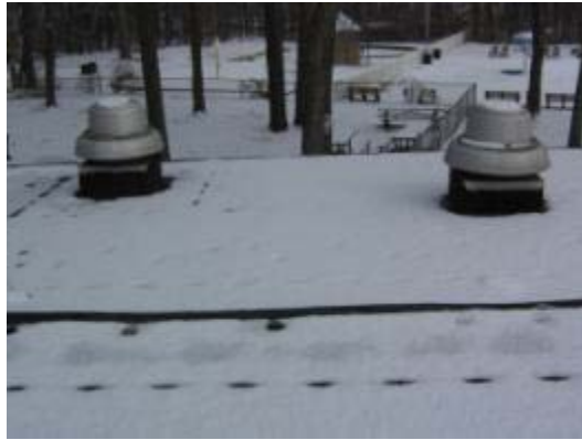
Rooftop Exhaust Fans
