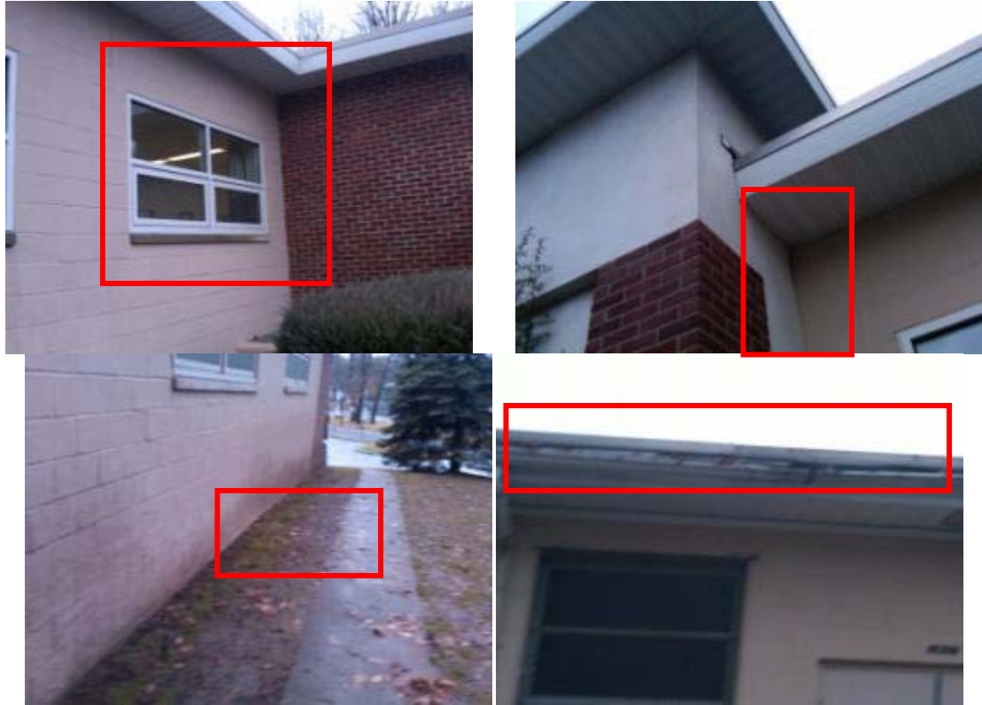
Signs of uncontrolled roof water runoff on walls due to missing/ defective roof flashing and missing gutters and downspouts as well as water damage at surface transitions, shifted concrete block and water damage due to poor site drainage.
