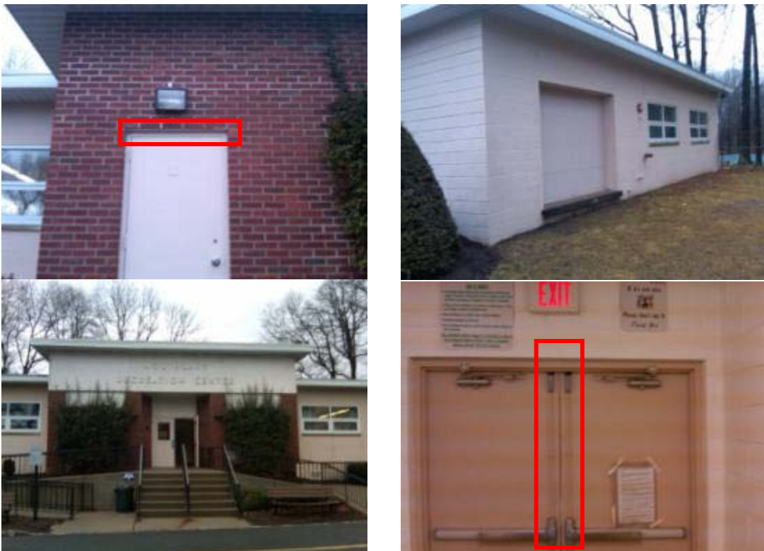
Examples of typical doors and problems such as deteriorated weather-stripping and exposed door lintels that are sources of thermal bridging.
