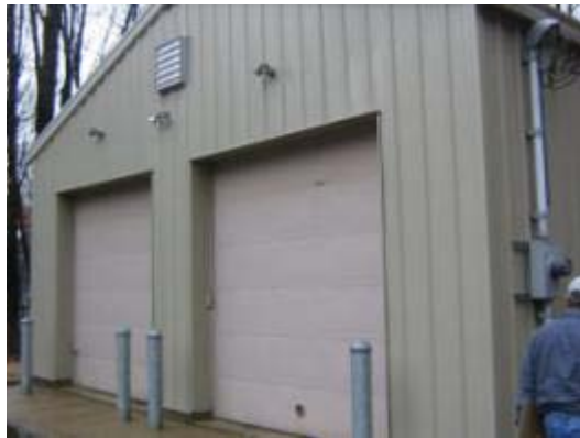
Exterior Halogen Fixture Above and Between Garage Doors
