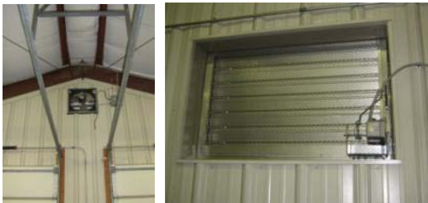
Exhaust fan in peak of structure, motorized louver in rear of space
