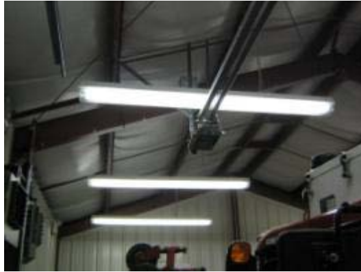
Interior Fluorescent Light Fixtures
