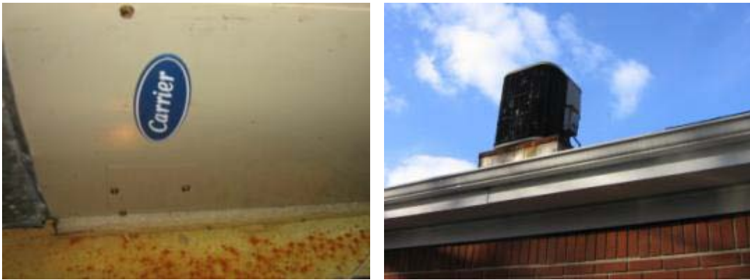
Photos – Air handling unit and paired condensing unit on roof
