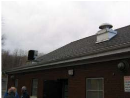
Sidewall and roof mounted exhaust fans serving the building
