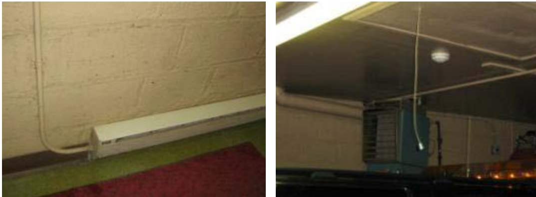
Electric baseboard heater, unit heater in garage
