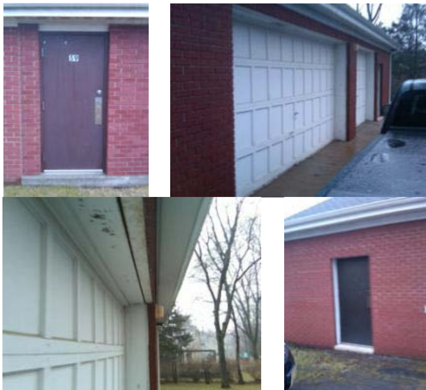
Exterior mold/ water damage signs on areas around doors and Damaged/ warped/ aged door frame
