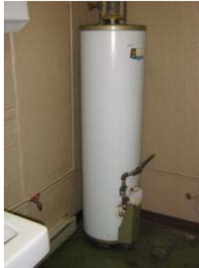
Photo – Domestic water heater
