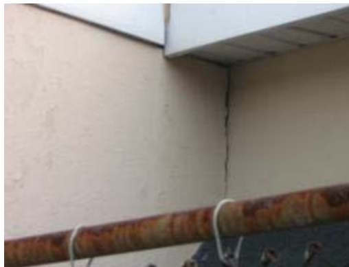
Large Crack Through Wall At Joint With Pool Building
