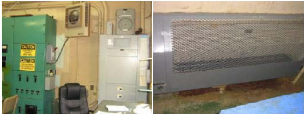
Electric Unit Heater In Deep Well (Left) and Electric Baseboard in Clear Well
