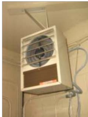
Photo – Electric Unit Heater (circa 1967) in Deep Well Building
