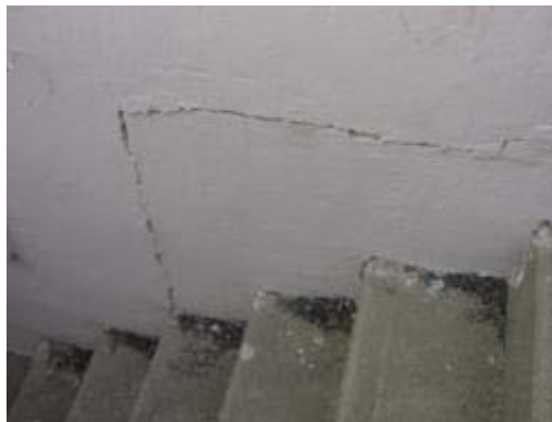
Deterioration Below Floor Line along East Wall of Deep Well
