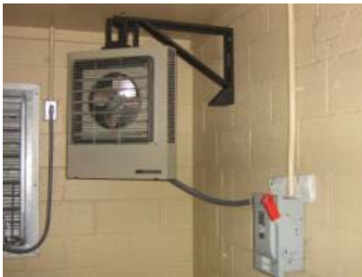
Electric Unit Heater
