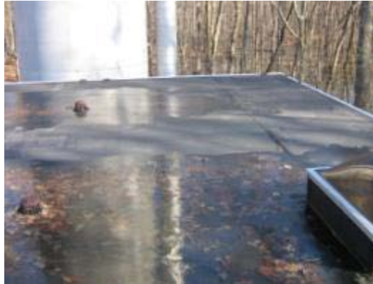
Water Pooling on Clear Well #2
