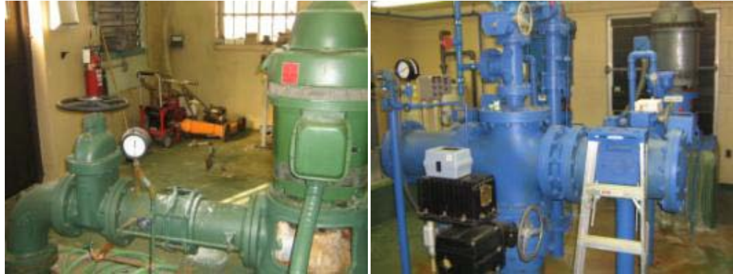
Deep Well Pump (Left) and Clear Well Pumps (Right)
