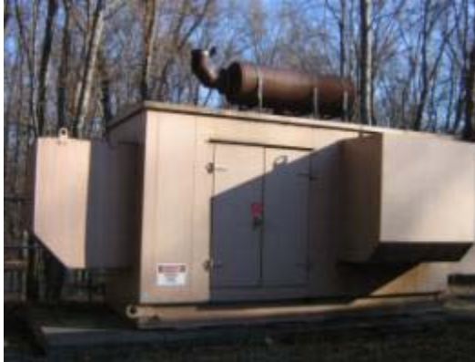
Emergency Generator at Well House #3
