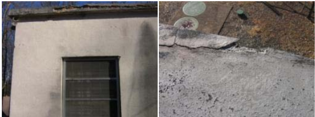
Deterioration of the coping on Deep Well #1
