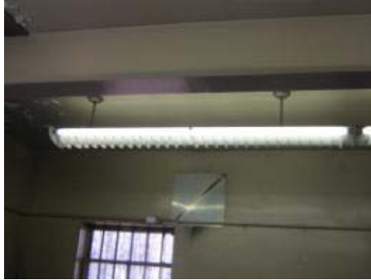
Suspended T12 Fluorescent Light Fixture
