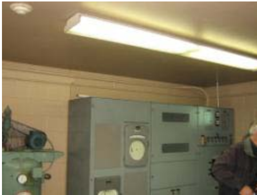
Surface-Mounted Fluorescent Light Fixture Above Pump Control Panel
