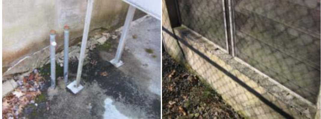
Serious deterioration of stucco on north and east sides of building
