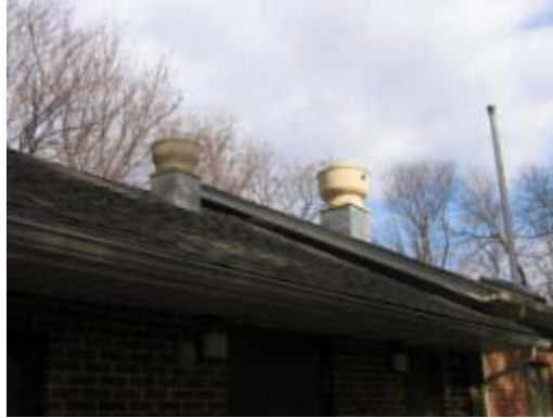
Rooftop Exhaust Fans
