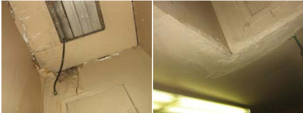
Typical water damage at the ceiling of the Deep Well building
