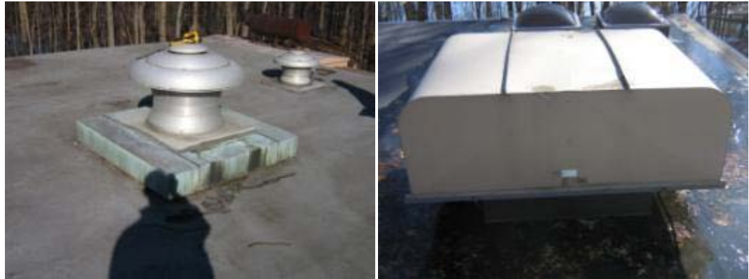
Rooftop Exhaust Fans for Deep Well (Left) and Clear Well Buildings
