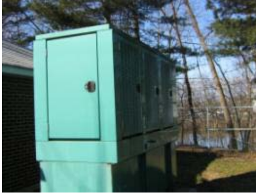
Diesel Generator at Well House #9
