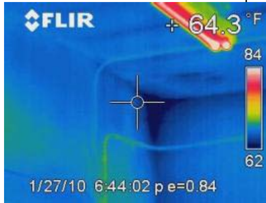
Infrared Image at Southwest Corner at Ceiling
