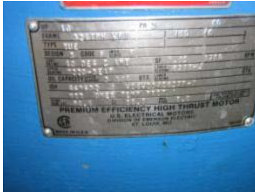
Clear Well Pump Nameplate
