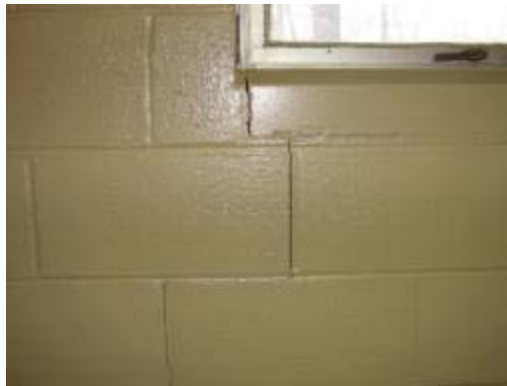
Through Wall Crack In Northwest Wall Of Deep Well
