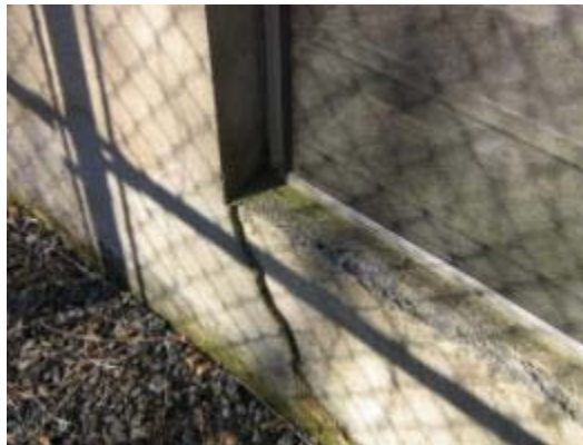
Serious deterioration of stucco on east side of building
