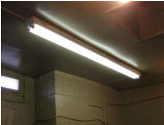
Surface-mounted fluorescent Light Fixture
