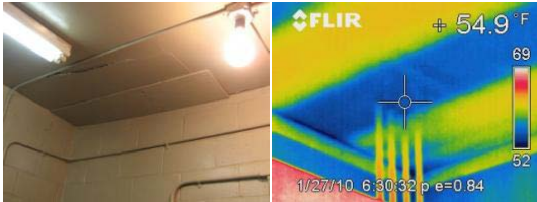
Digital Photo and Infrared Image of Plywood Panel
