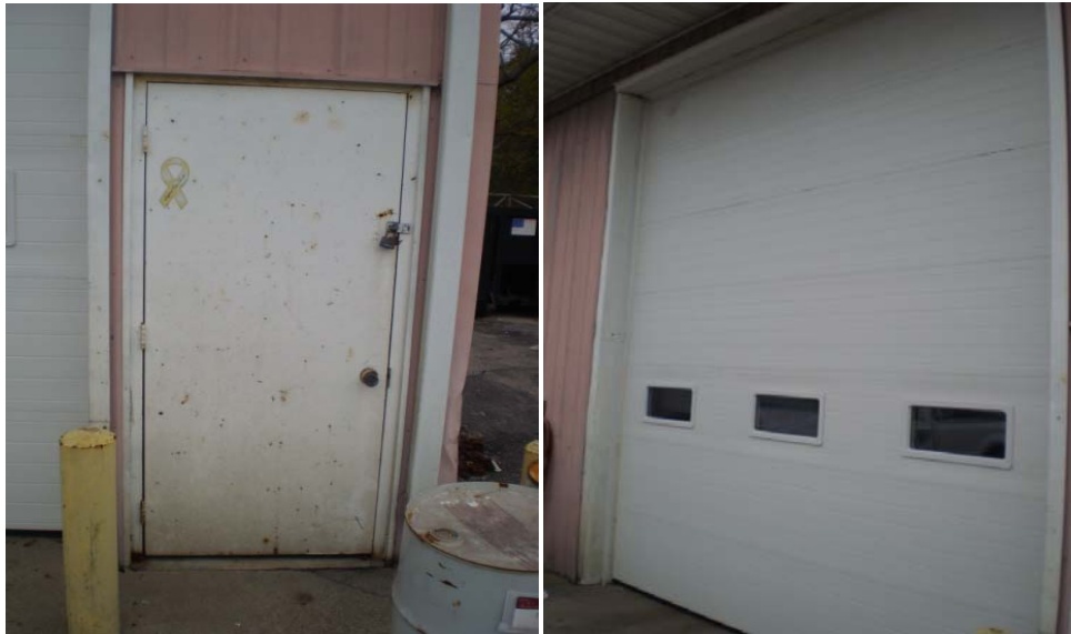
Missing/ worn weather stripping and damaged/ warped/ aged door frame
