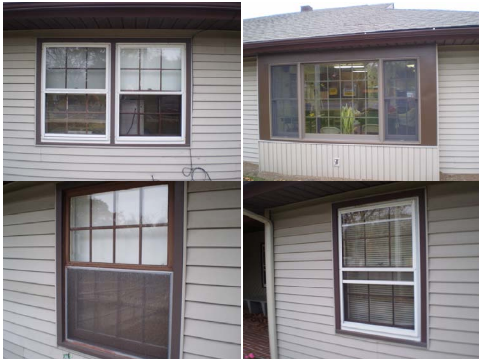
Typically installed windows with wooden frame unit showing signs of advanced age and some damage to the frame.
