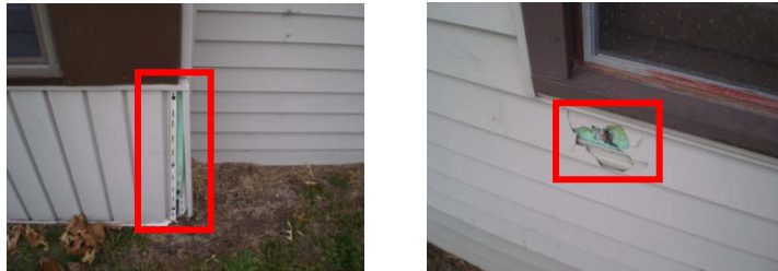
Damaged exterior wall finishes with missing vinyl siding to be replaced
