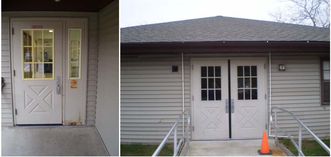
Exterior doors exhibiting worn weather stripping and damaged door frame
