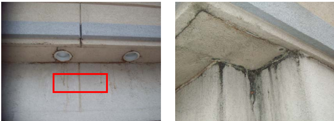
Signs of water damage at perimeter walls due to missing/ineffective site drainage
