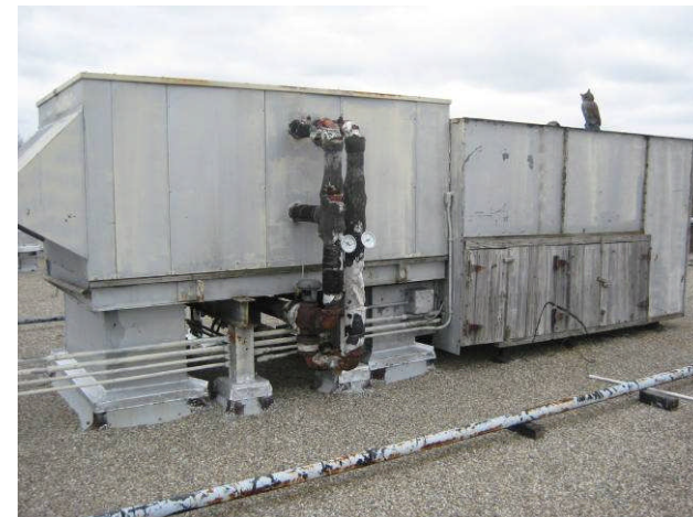
Pool HV unit w/ electric heating coil and heat recovery coil
