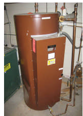
Picture: Maintenance Building Electric Hot Water Heater
