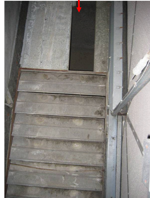
PHOTO: PE – HV-1 & EF 8-1 Energy Recover System
