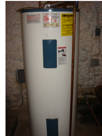
Administration Building: Electric Hot Water Heater
