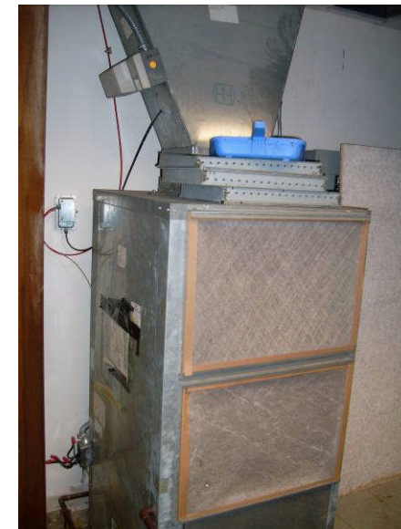
Pictured: Typical WSHP Serving Classrooms
