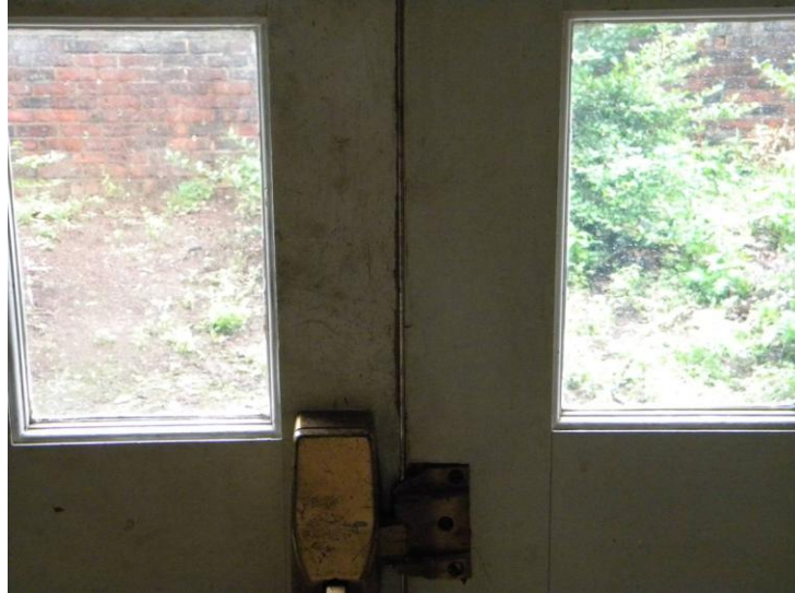
Daylight can be seen between two emergency egress doors at old section
