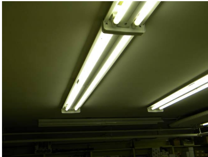
T12 Fluorescent Lamps in Processing Room
