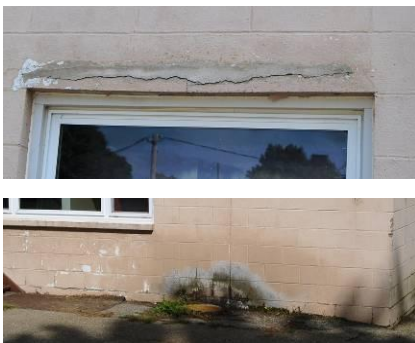
Condensate Drip Damage
