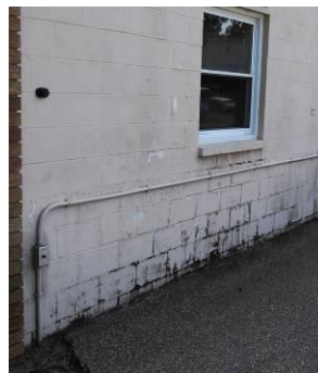
Roof Water Runoff Damage
