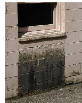
Excessive Algae Growth under Window
