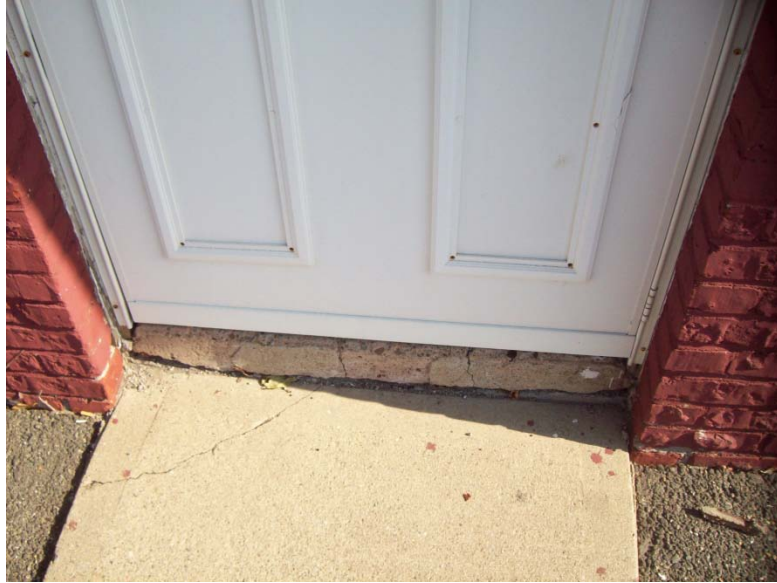
Cracked Building Base
