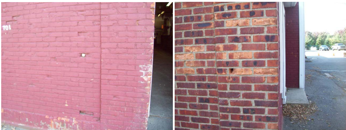
Instances of Damaged Masonry Units
