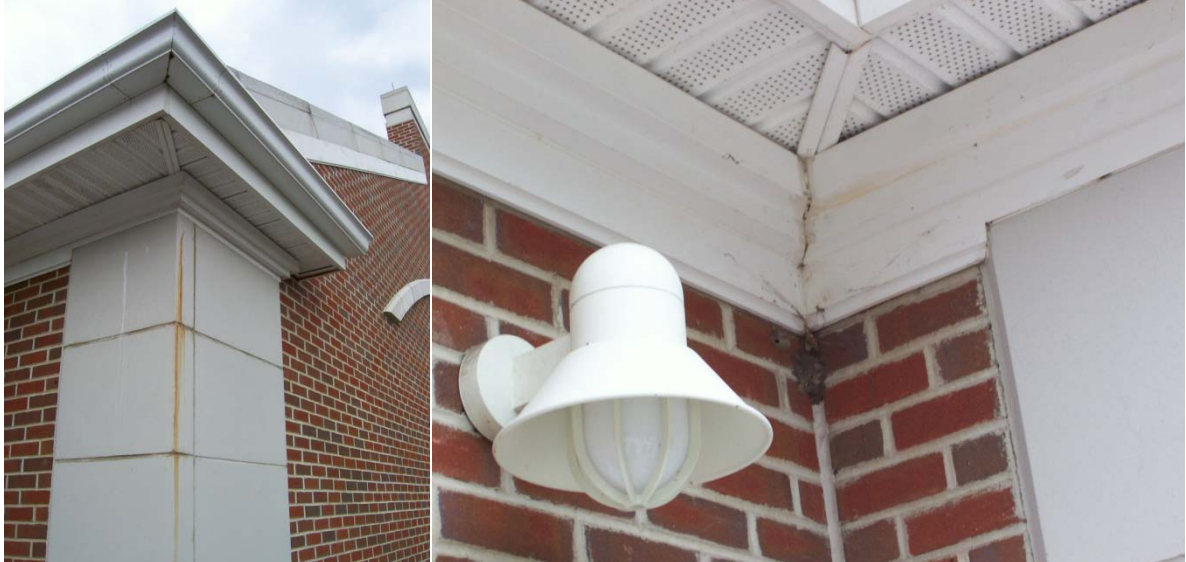
Exterior wall cracks and water damage at corners and surface transitions
