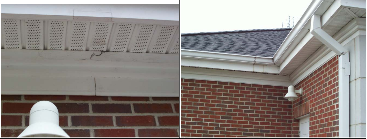
Example of damaged roofing eave
