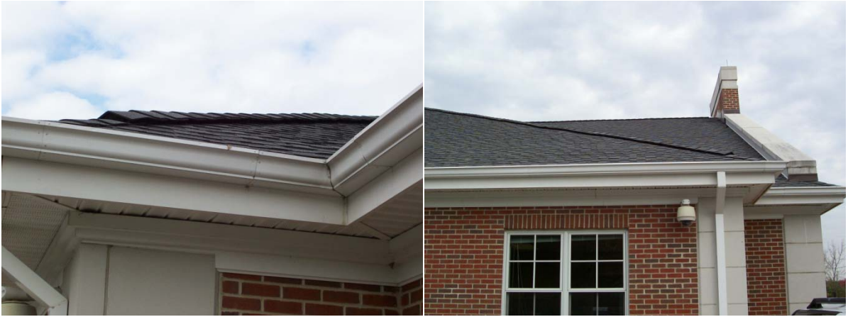
Example of uprooted shingles
