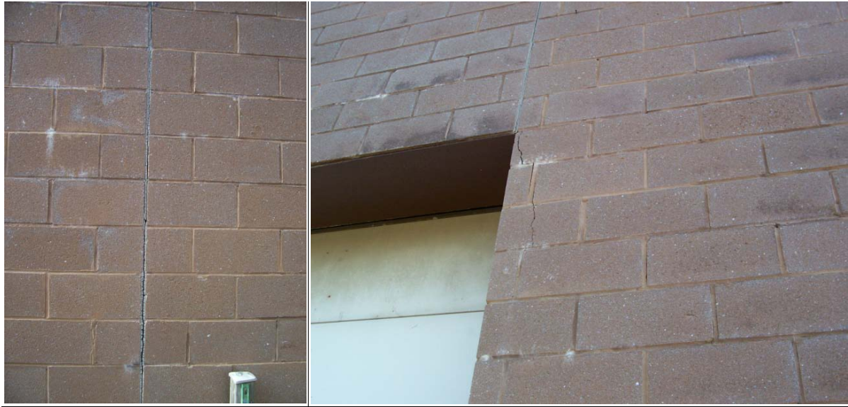
Exterior wall cracks at seams and cracked concrete blocks
