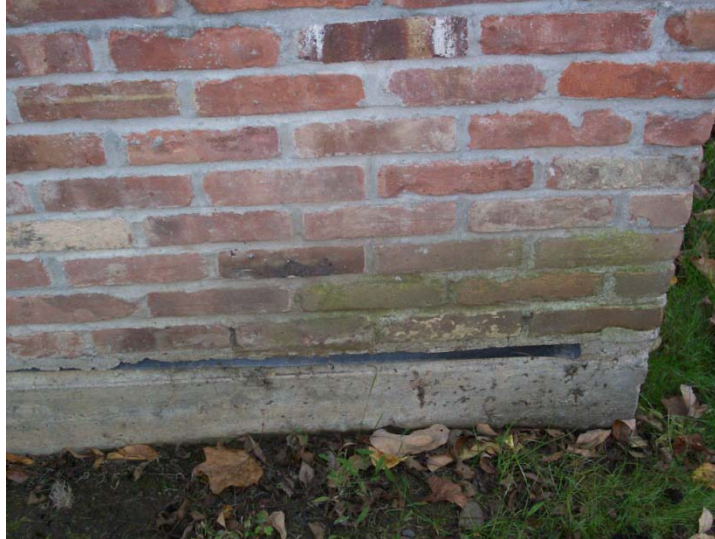
Exterior wall with water damage and cracked seam at base transition
