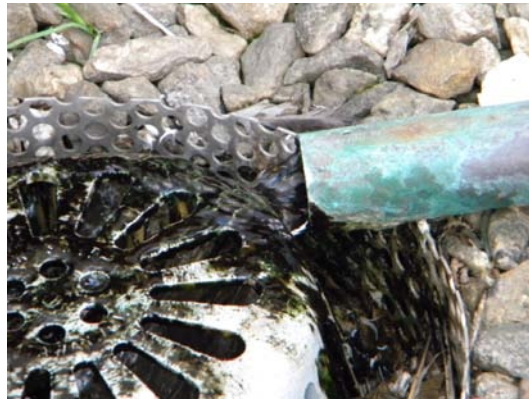
Image showing cooling tower water draining continuously when cooling tower is in operation.
