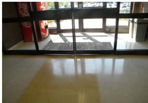
Example of air gaps and missing weather-stripping of entry and vestibule doors.
