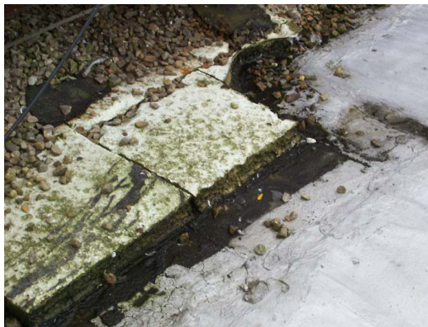
Built-up roof section showing damaged insulation
