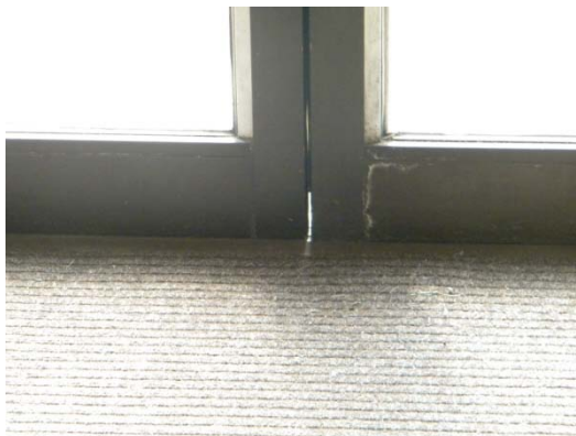
Example of air gap and missing weather-stripping at entry door
