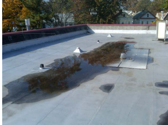
Built-up roof section above the garage showing signs pooling
