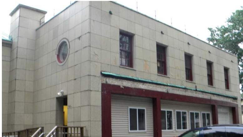
Example of damaged tile in the rear of the building
