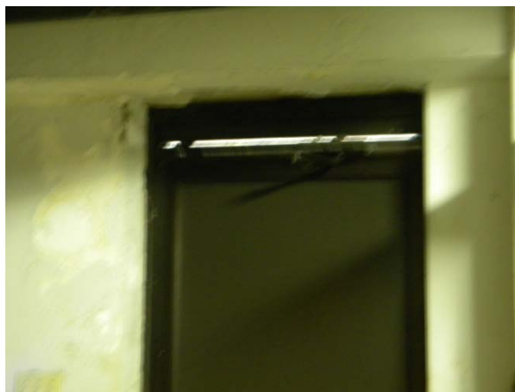
Air gap at fiberglass door
