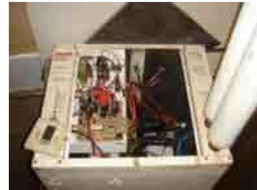
Picture: Tillis Hall Heat Pump
