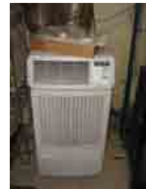
Picture: Server Room AC Unit set for 63 °F
