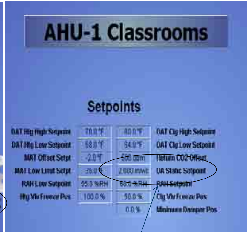
Picture: Davidow Hall – Static Pressure Setpoint locked at 2.00 in/w.c.
