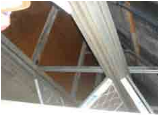
Picture: Davidow Hall - AHU – 4
