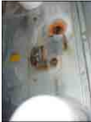
Picture: Davidow AHU -1
