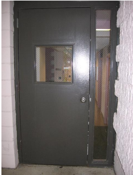
Worn weather-stripping at side door
