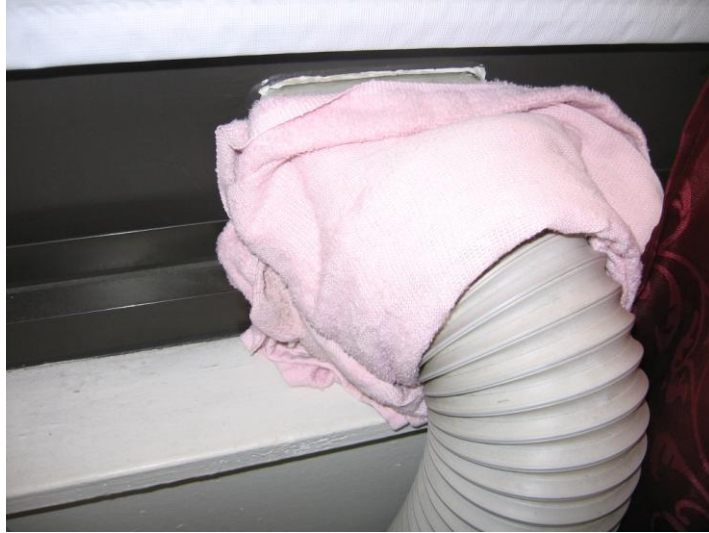
Stand alone air conditioner ducted through an apartment window
