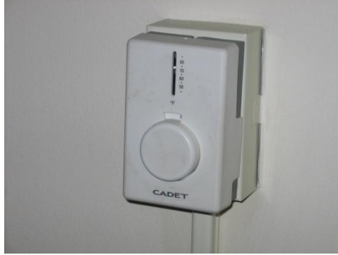
Typical thermostat for electric baseboard
