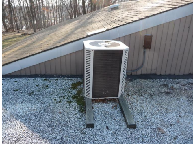
Lounge / bar rooftop condenser
