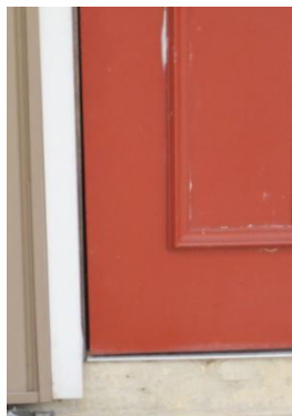
Missing / worn weather stripping
