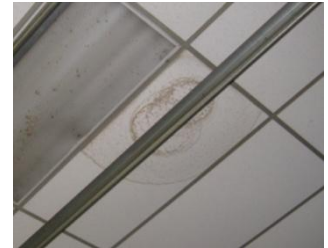
Signs of mold / water damage on interior finishes
