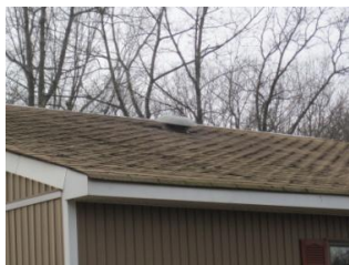
The roofing material has reached the end of its useful lifespan.
