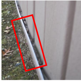
Faulty construction detail at vinyl panel termination that can promote water / moisture penetration into the wall cavity by clogging or wind driven rain.
