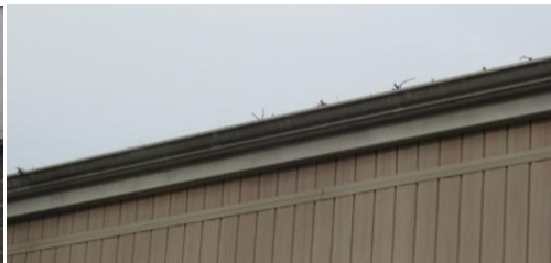
Clogged/ ineffective gutters
