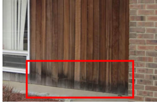
Signs of water damage at perimeter walls due to missing / ineffective site drainage.
