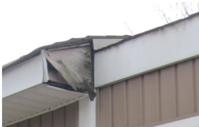
Missing / deteriorating wood trim / moldings
