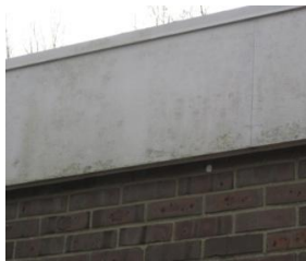
Missing / deteriorating wood trim / moldings
