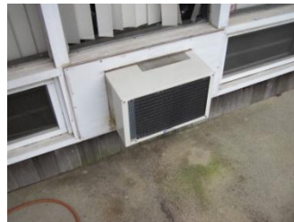
Air-leakage at sleeved window / wall air-conditioning units
