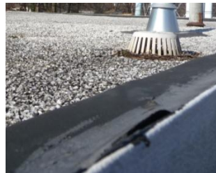
Delaminating roof membrane / patches
