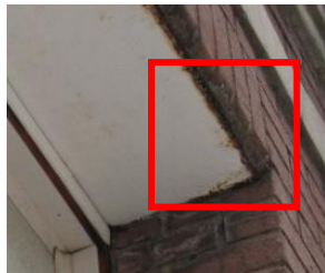
Rusted / deteriorated steel lintel.
