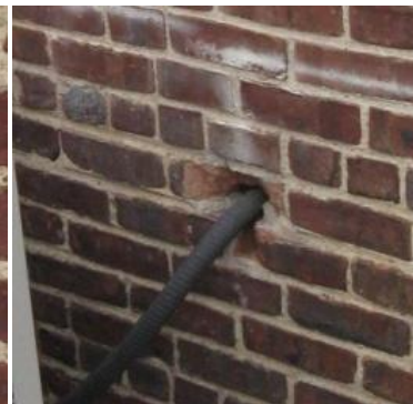
Un-caulked / unsealed exterior wall penetrations
