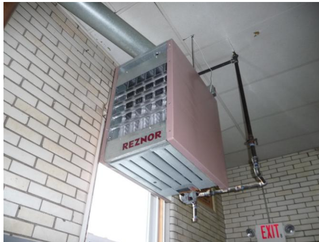
Truck bay Reznor gas heaters
