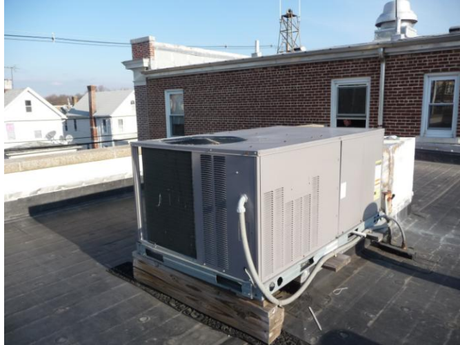
Lounge / bar rooftop Carrier heat pump
