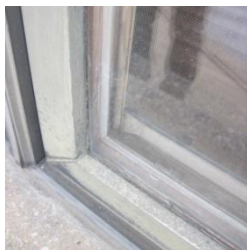
Single glazed window with ineffective frame
