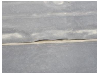
Delaminating roof membrane / patches
