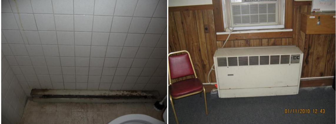
Rusted and old wall electric coil heating emitters
