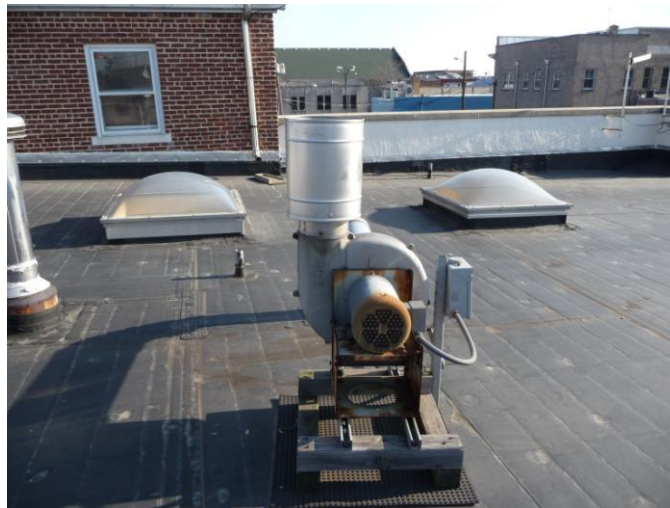
Rooftop fan to vent fire truck exhaust
