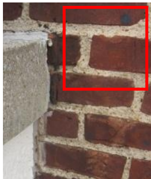
Deteriorated mortar joints
