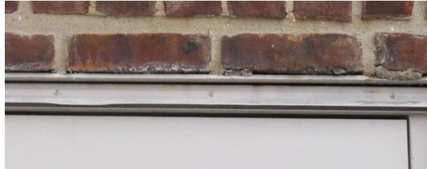
Cracked / deteriorated mortar joints
