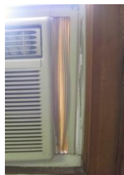
Air-leakage at sleeved window / wall air-conditioning units
