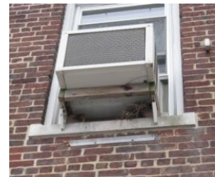
Air-leakage at sleeved window / wall air-conditioning units
