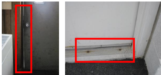
Missing / worn weather stripping
