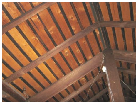
Missing soffit and ridge vent system
