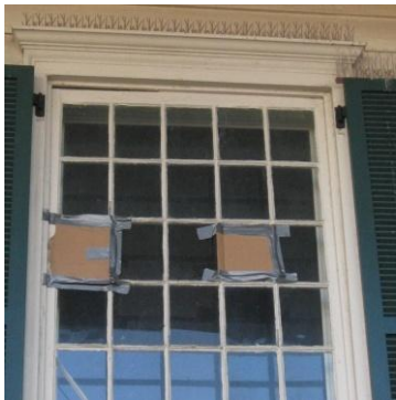
Broken / missing glazing
