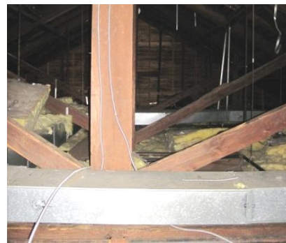
Uneven / ineffective attic insulation found.
