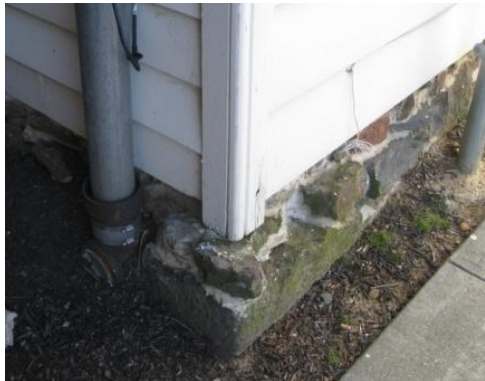
Missing cap flashing for exposed foundation wall.
