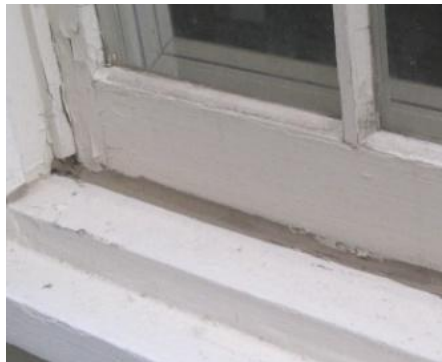
Damaged / aged window frame
