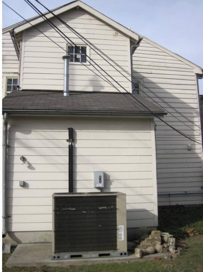
Condenser in back of the furnace / evaporator attached enclosure
