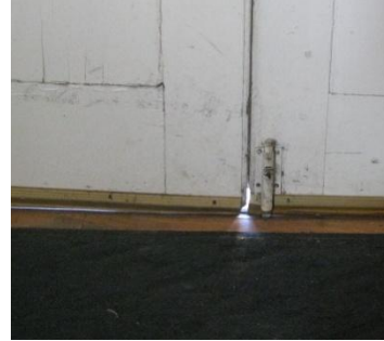
Missing / worn weather stripping
