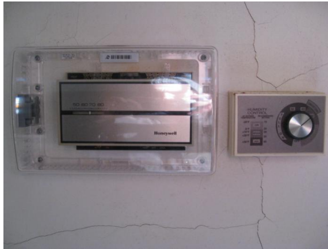
War Memorial building wall mounted programmable thermostat and humidity controller
