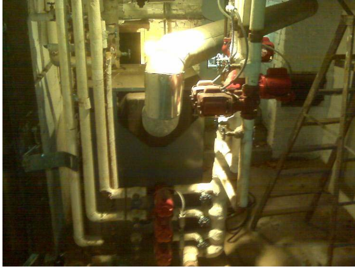
The boiler in the center of the picture provides heat and domestic hot water.
