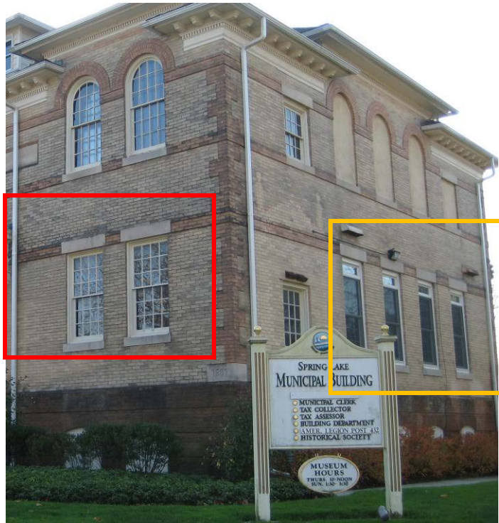
Red box highlights older single pane windows. Orange box outlines newer double pane windows
