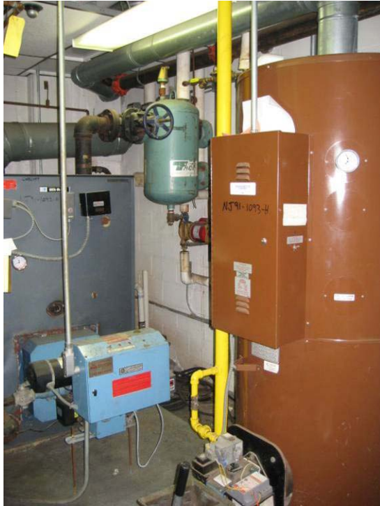
A.O. Smith Water Heater to be replaced
