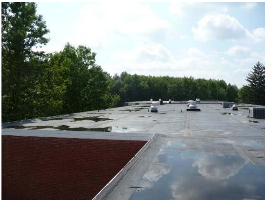
Pooling on Roof
