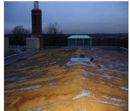
High School Foam Roof Deterioration
