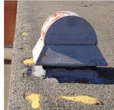
Deteriorating Foam Roof
