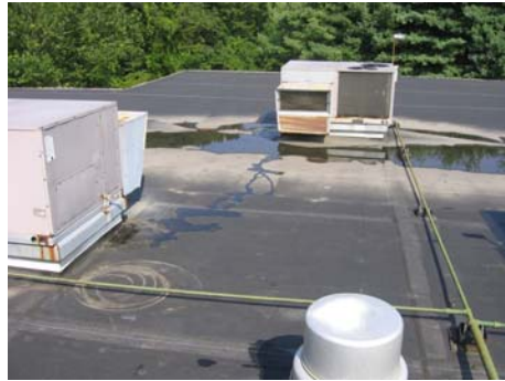
Pooling on older roof section
