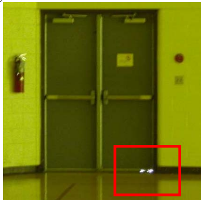
Worn or missing weather-stripping in gymnasium
