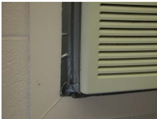
Wall AC sleeve unit seal shows insufficient air sealing
