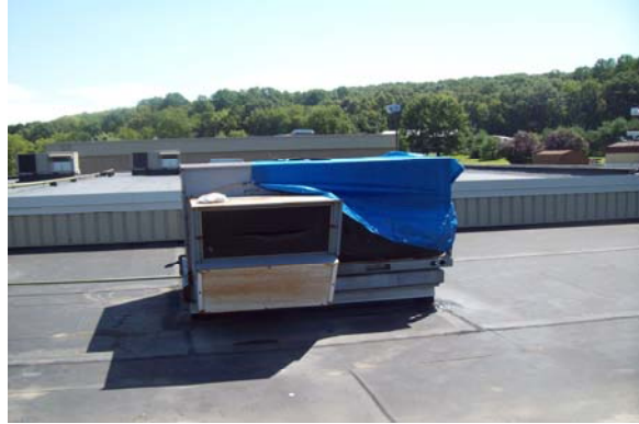
Rooftop unit shut-off and covered with a tarp
