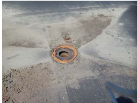
Drain missing screen and allowing debris to gather on roof
