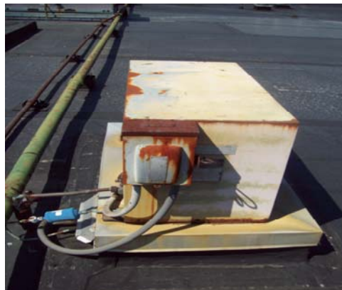
De-commissioned condensing unit
