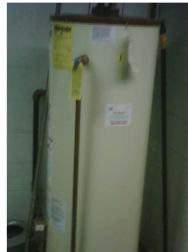
Town Hall building’s water heater
