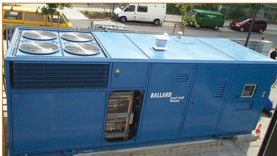
figure 4. A 250-kW natural-gas-fueled PEM fuel cell stationary power generator.
