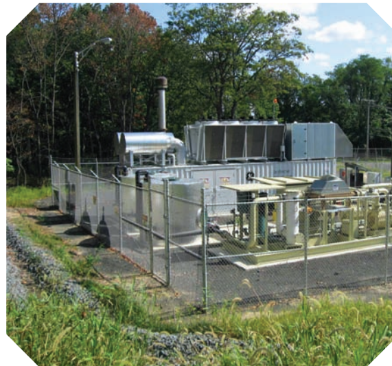
Monmouth County's one megawatt sustainable biopower project produces enough energy to support their materials processing and recovering facility.
