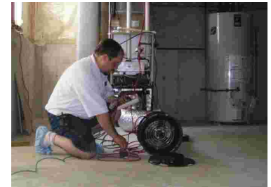
A properly installed and tested duct system maximizes your heating/cooling system efficiency.
