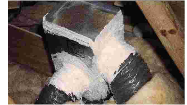
Contractors use a special mastic & fiberglass perma-sealant to guard against air leaks in the duct system.
