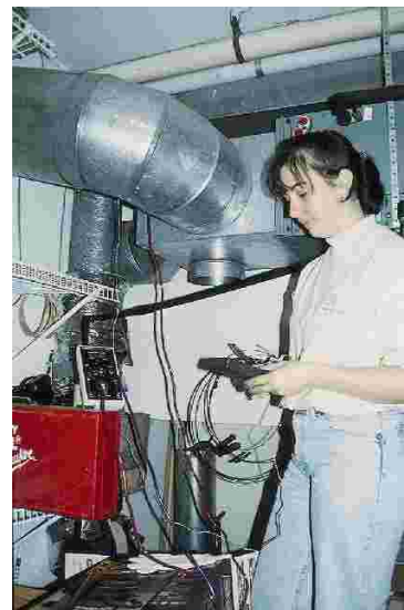
Computerized Air Flow Testing
