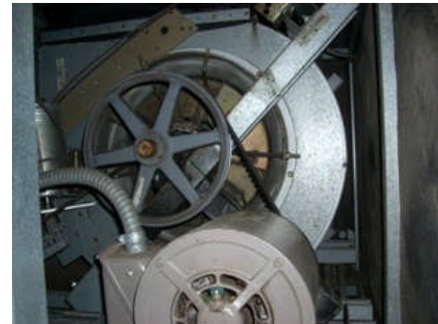
Air Handling Unit w/ Vortex Dampers
