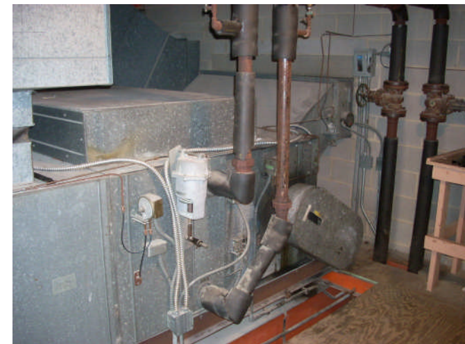
Pool HV unit w/ hot water heating coil
