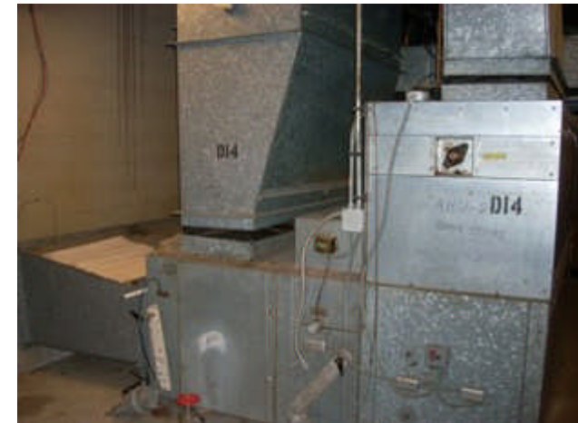
Air Handler Unit in D-Block of Lewis Parker Bldg.
