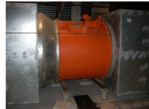
AHU-1 Return Fan in Library
