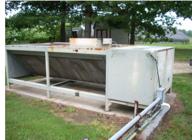
Air-Cooled Reciprocating Chiller - 800 Building
