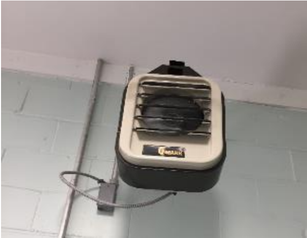
Image 2 Main Building electric heater
