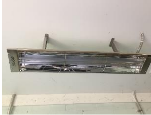
Image 3 Well #2 and Generator bldg. electric heater
