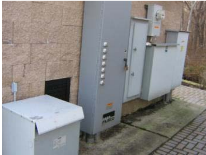
Photo – Musco Lighting Controller for Sports Field Lighting
