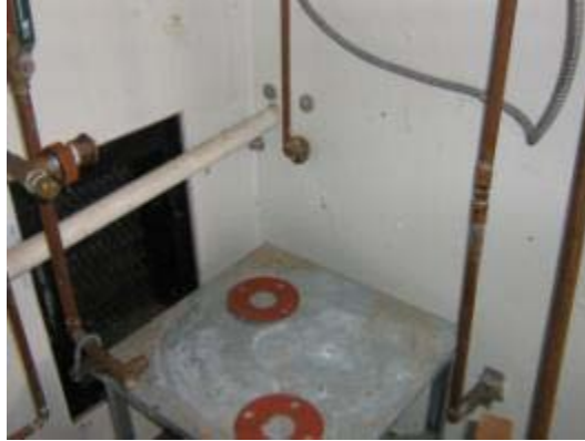
Platform Where Domestic Water Heater Is Located During Operational Hours
