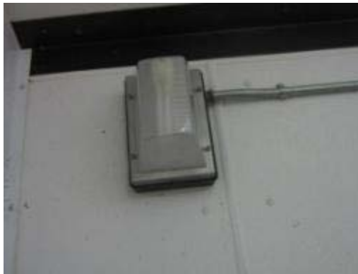
Photo – Light Fixture With Compact Fluorescent Lamp in Toilet Room
