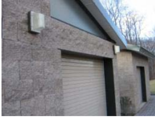
Photo – Exterior Metal Halide Fixtures
