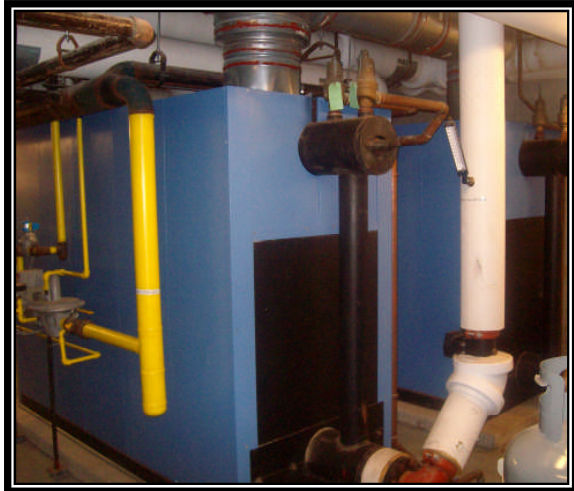
An Existing Ross School Boiler
