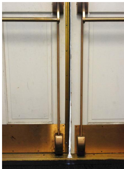
Missing or Worn Weather-Stripping at front door
