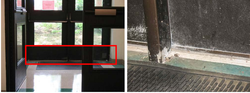
Double doors in good condition, in need of weather-stripping
