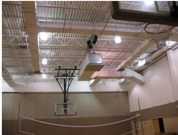
Gymnasium Metal Halide lighting
